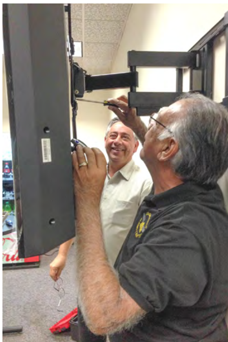
Eddie Dunn and Andy Vaquera installing a flat panel TV at the Enlisted Aircrew Student Breakroom at CEA/CoE, 344th Training Squadron, Lackland AFB TX
